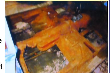
Holes in the floor board
